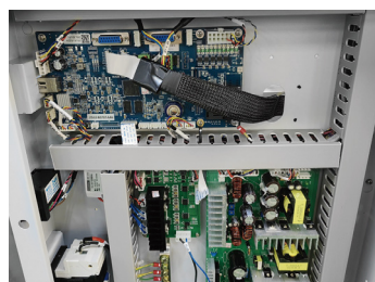
Hoson Board and Control System
